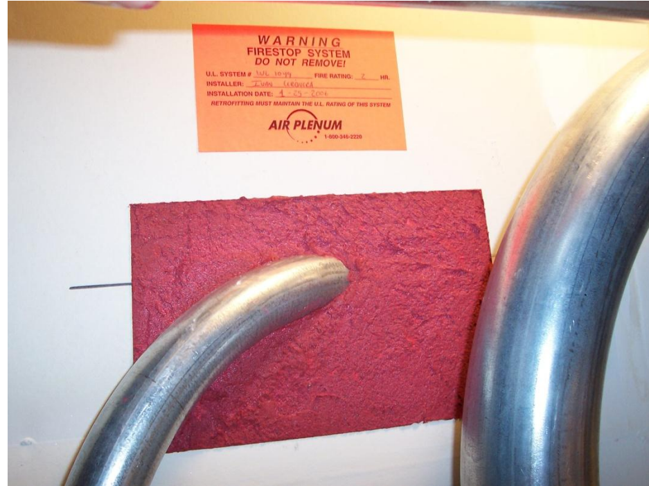
After – By Air Plenum
