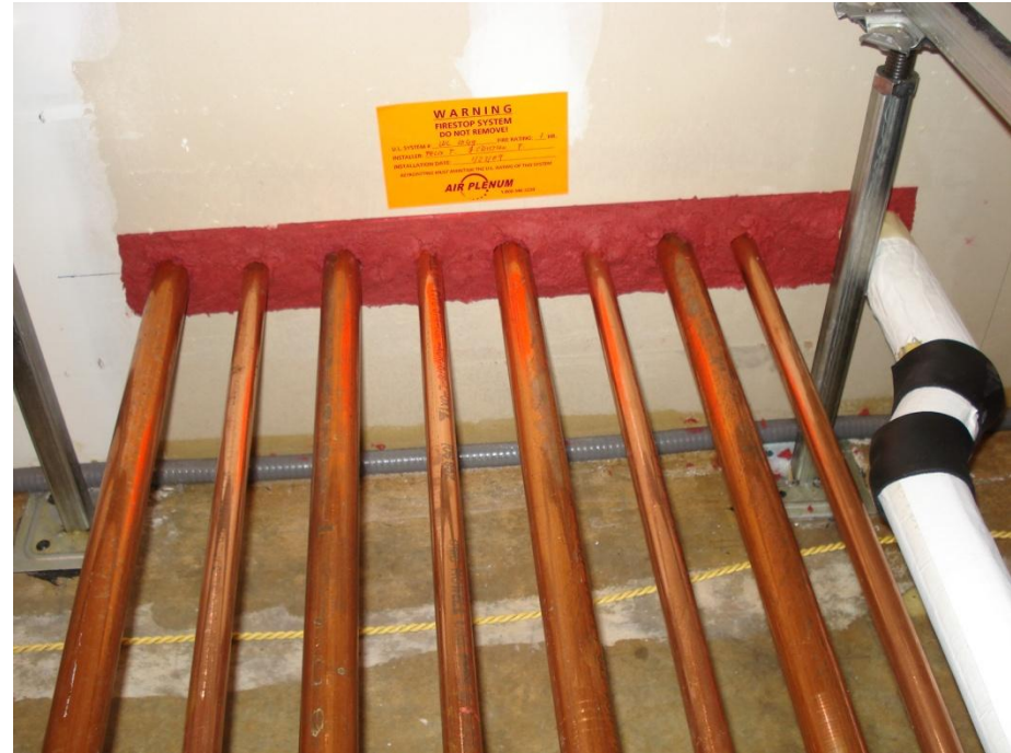
After – By Air Plenum
