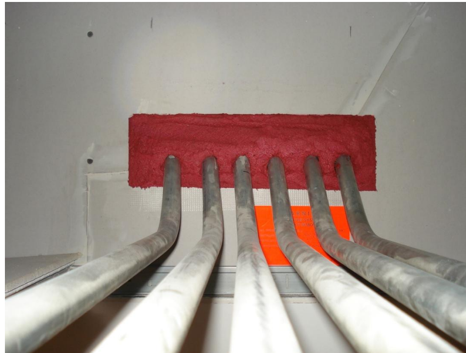
After – By Air Plenum
