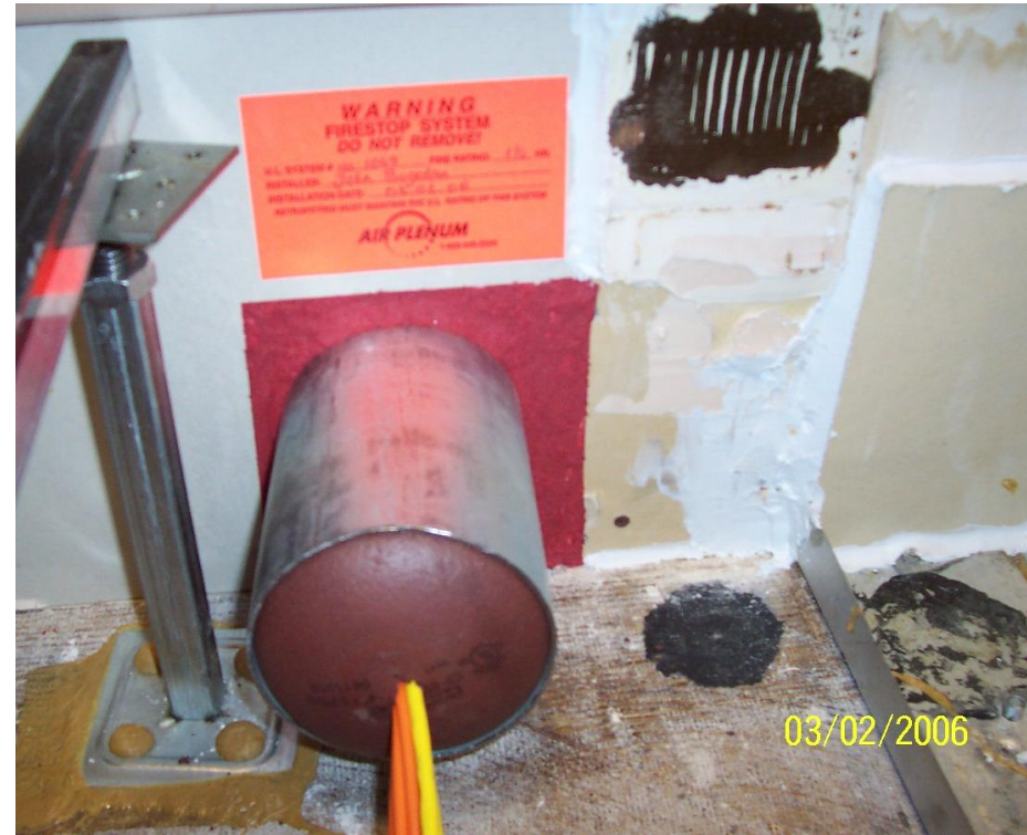
After – By Air Plenum
