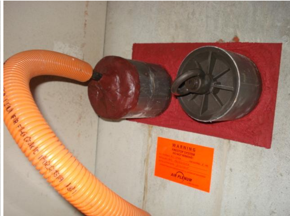
After – By Air Plenum
